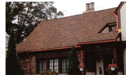
■ Eurocraft copper gutters, downspouts, and flashing were installed on this New York residence five years ago. They were coated with Permalac, a clearcoat lacquer, to prevent oxidation. Photos courtesy of Peacock labs.
